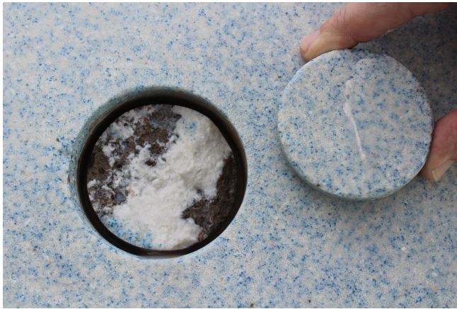
Figure oB-00058 – Core 4 with Nodule Following Crack and Bond Failure
