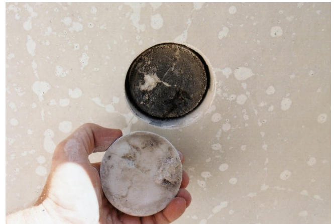
Figure oB-00015a – Bond Failure and Cavity Behind Crack and Nodule
