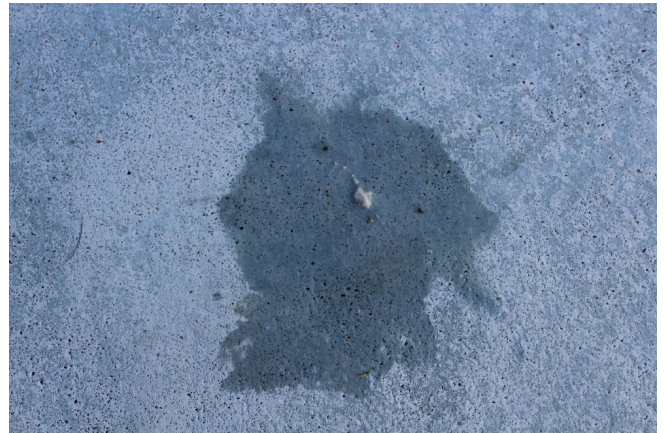
Figure oB-00060b – Close-up of Nodule on Microcrack With Leaking Water
