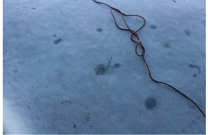
Figure oB-00060a – Pool Floor with Nodules Over Cracks and Sub-Surface Trapped Water
